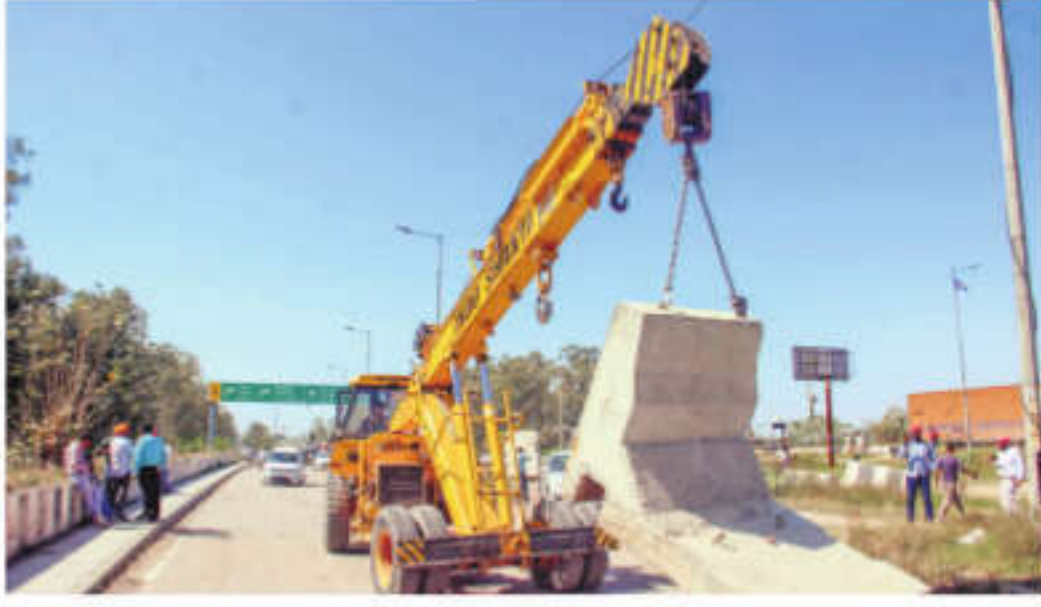
Concrete barricades being removed after the eviction of agitating farmers from the Shambhu border, in Patiala district on Thursday | PTI
